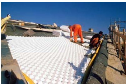
Installation of the drainage element Floraset® FS 75 on the pitched green roof area.
